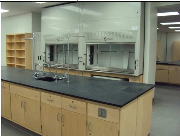
New fume hoods
